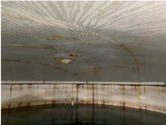
Water Chamber Roof - Coating failures or issues Photo
