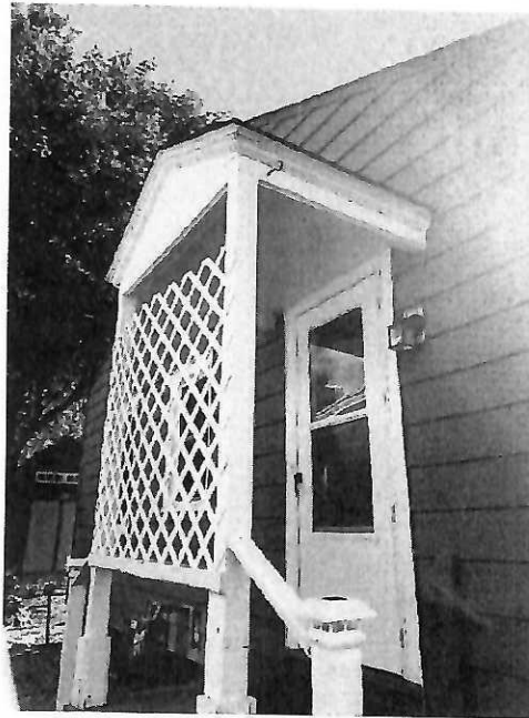
Existing Side Entry that is over the required side setback
