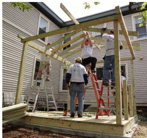
Rotary volunteers working for Rebuilding Together constructing a gazebo for the veteran’s home on Church Ave.
